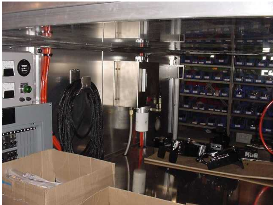
Oil Reservoir Tank (Photo 2)
